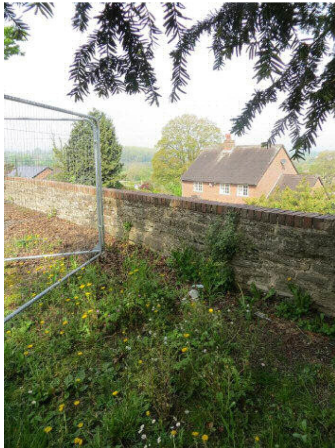
Photograph 5: Wall above churchyard ground level with brick on edge coping (2018)
