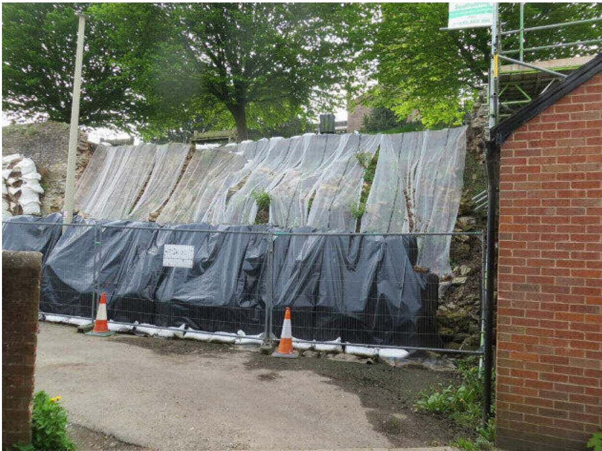
Photograph 8: Area of collapse with protection over and ballast bags as barrier (2018)
