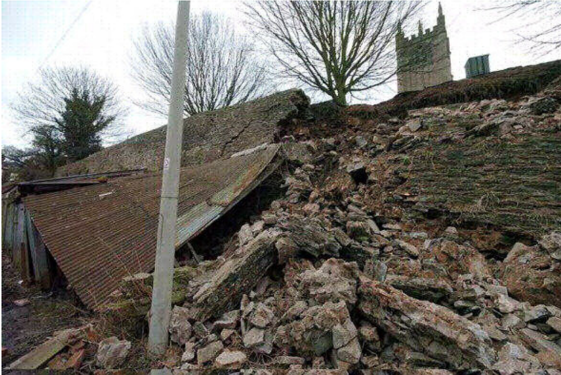
Plate 14 Collapsed wall in 2013 (Shropshire Star)
