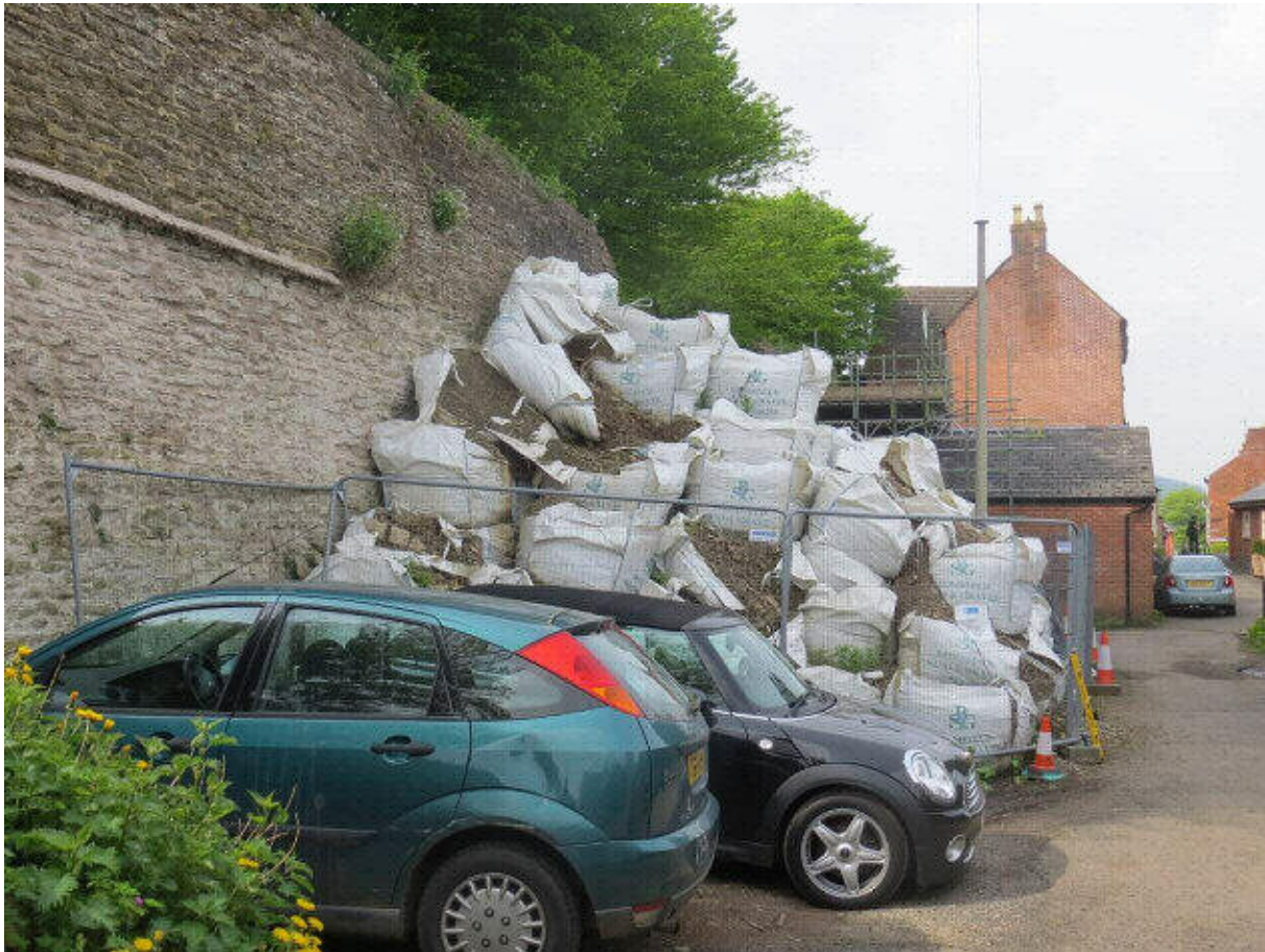
Photograph 9: Ballast bag buttress to east end of collapsed section (2018)
