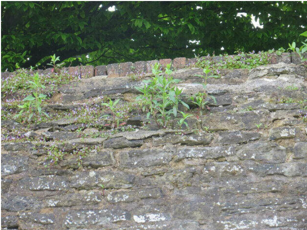
Photograph 16: Wall outside courtyard better consolidated but may be cement based mortars. Plant growth still obvious suggesting water paths within the walling.(2018)
