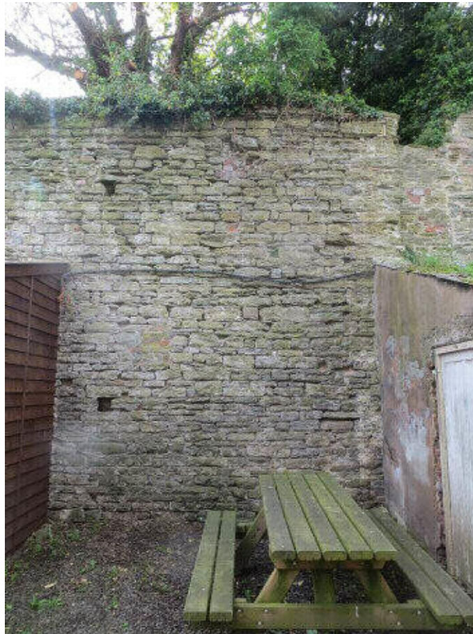
Photograph 15: Open nature of jointing within Compasses courtyard area (2018)
