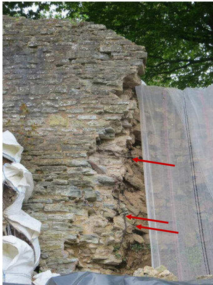
Photograph 17: Roots seen in wall width (2018)
