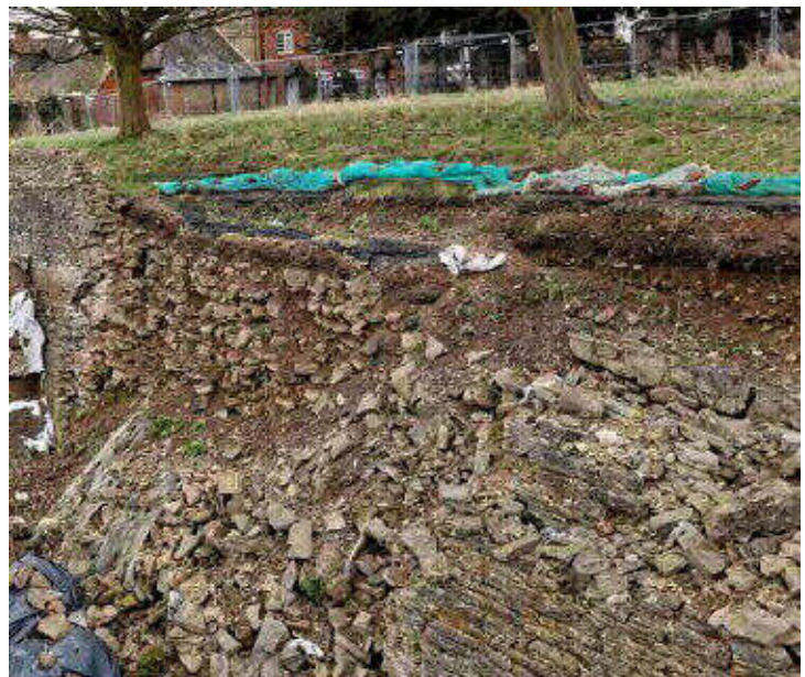
Plate 19 Area of collapsed walling, looking east (James Brennan Associates)
