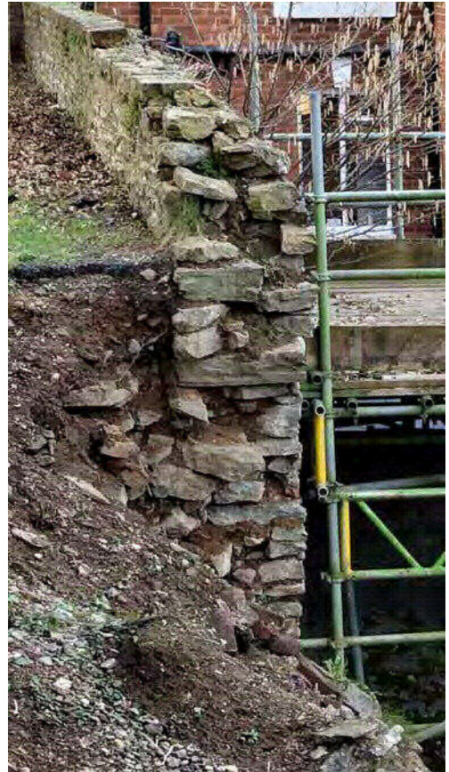
Plate 18 Section of the wall exposed to the west of the collapse (James Brennan Associates)
